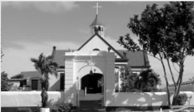
On St. Croix, a crew recently painted St. Ann Church and its surrounding walls.
